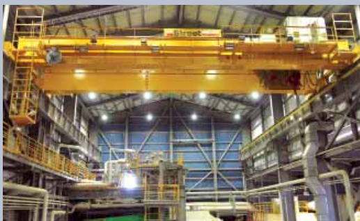
87t Power station crane
